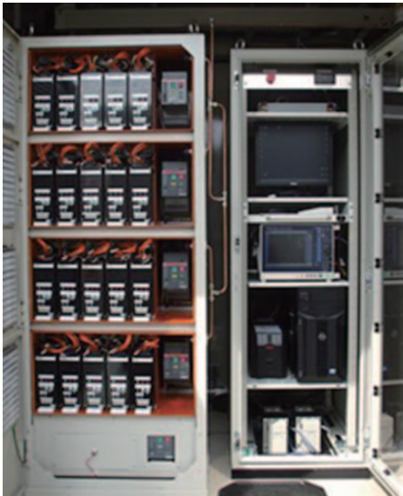
図7 25kWh 蓄電システムの外観 Fig.7 Appearance of 25kWh-energy storage system (ESS)
