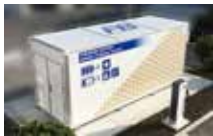
ESS (Energy Storage System)
